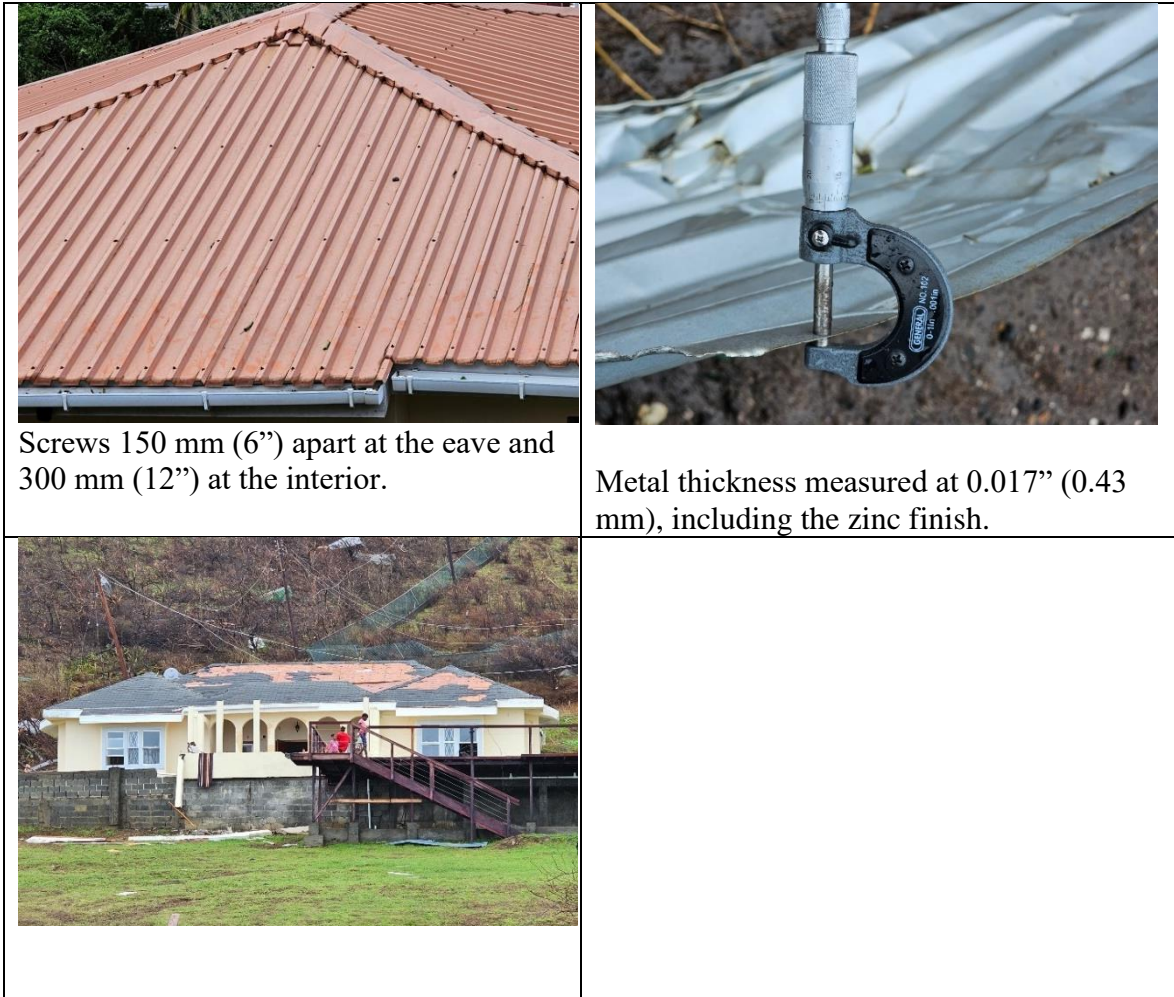
Figure 7 – Roof cladding failure modes.
