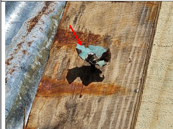
Ripped cladding – remaining on the screw.
