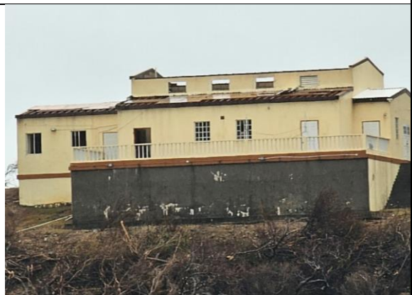
Full cladding and frame loss over highest roof in church.
