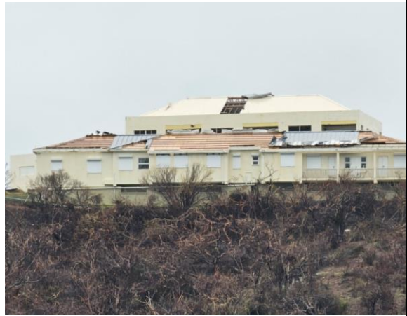
Hospital with partial cladding loss.
