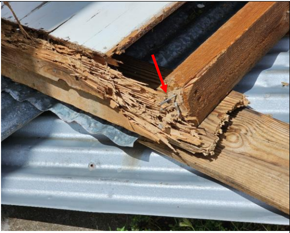
Rafter nailed to termite damaged wall beam.
