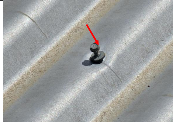
Screw pulling out of timber frame.
