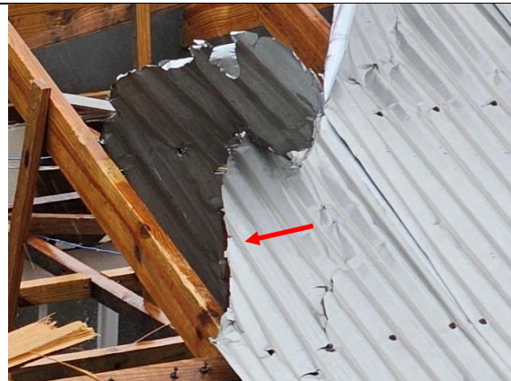
Torn roof cladding.
