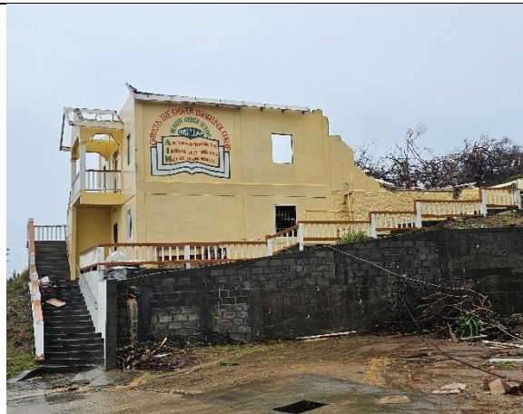
Damage to church. Failure likely by movement of the roof frame transferring lateral forces to the walls.
