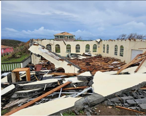
Church with unreinforced masonry walls and without adequate shear walls. Failure likely by movement of the roof truss transferring lateral forces to the walls.
