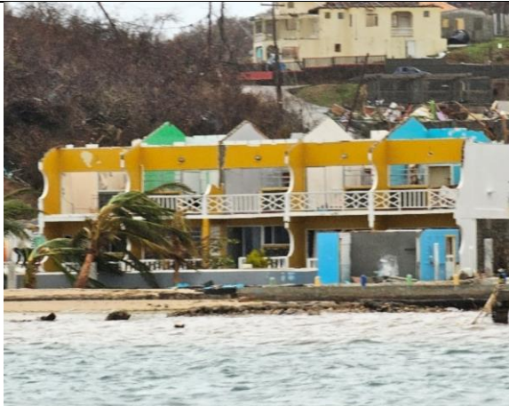
Hotel accommodations, with full cladding and roof frame loss.
