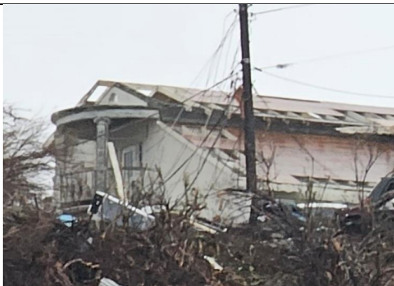
Cladding loss and partial frame loss of church.
