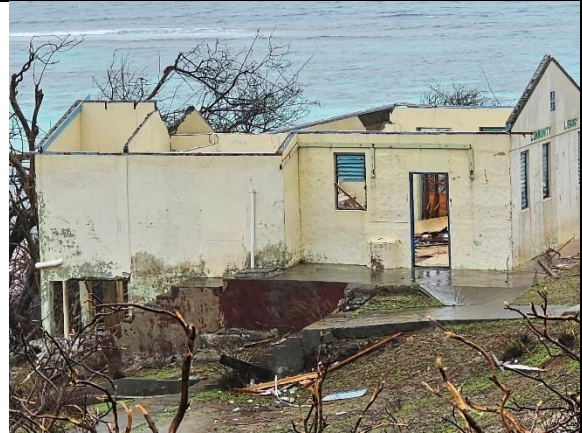
Full roof cladding and frame loss of library.
