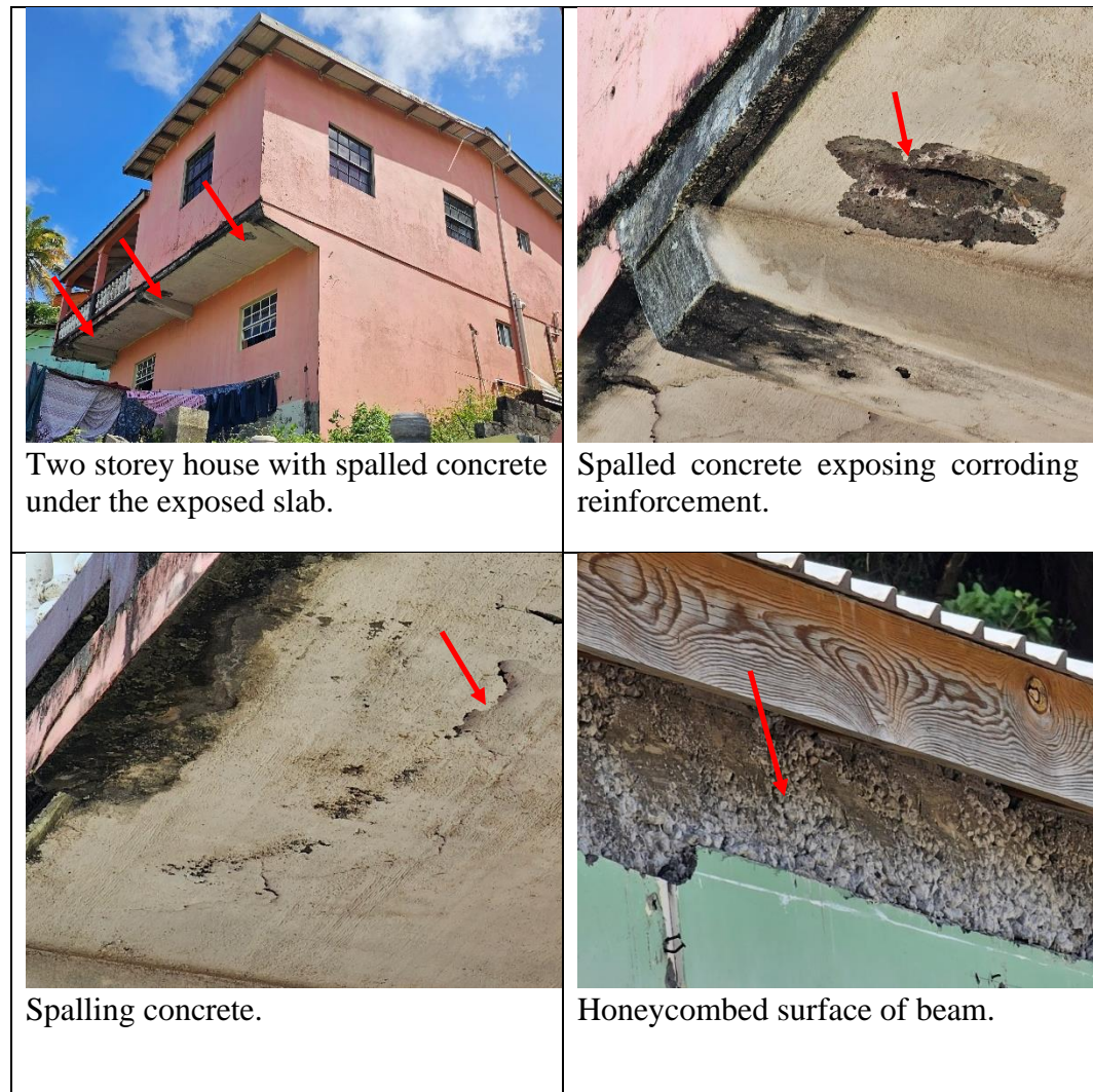
Figure 11 – Spalling and honeycombed concrete.
