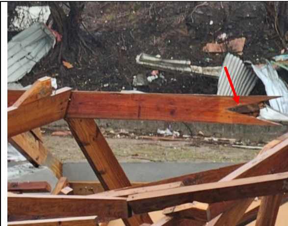
Likely point of failure – the joints in the ridge beam.
