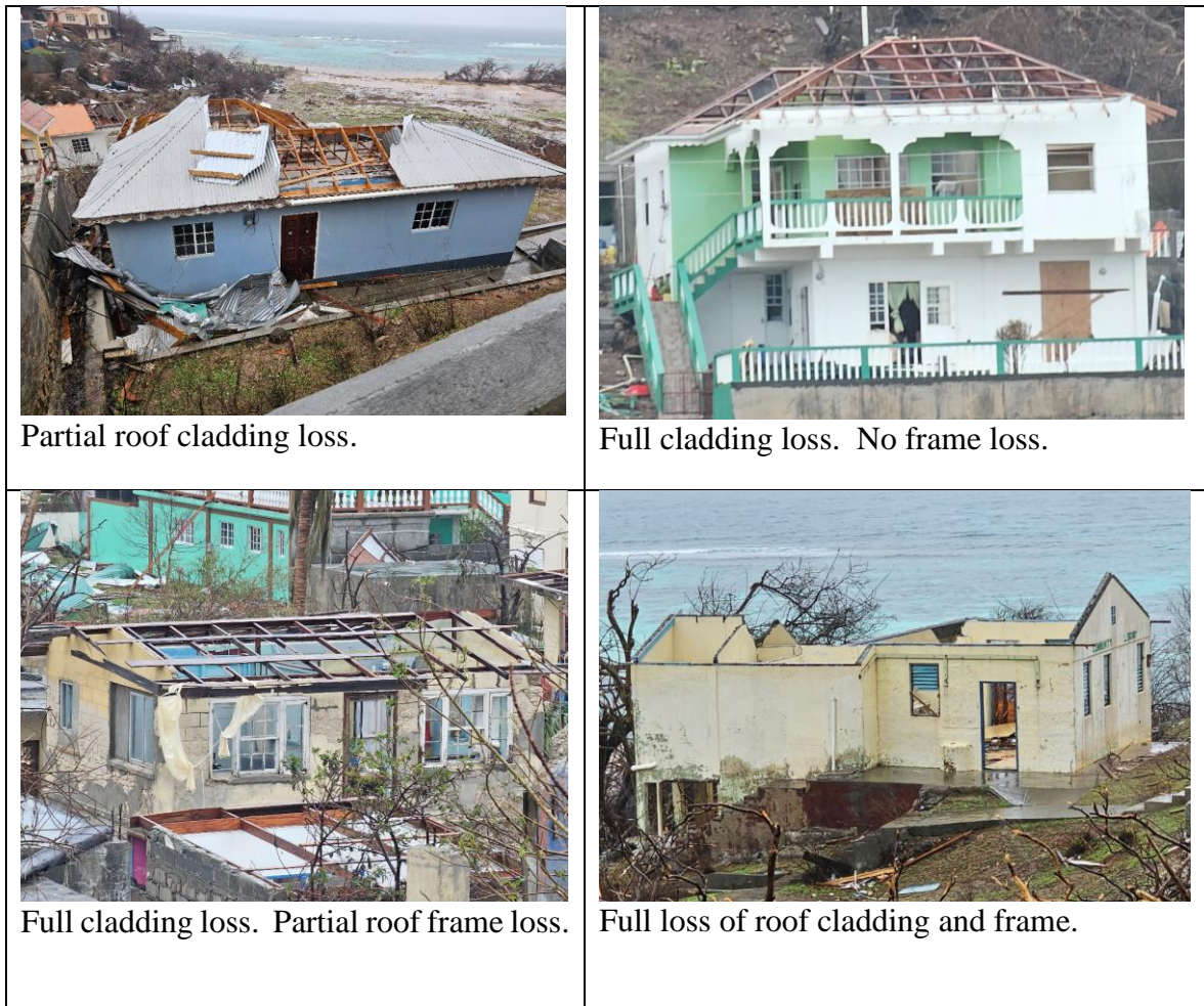
Figure 2- Examples of roof cladding and frame losses.
