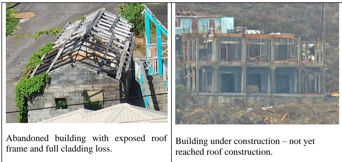
Figure 5 – Examples of erroneous apparent roof loss.
