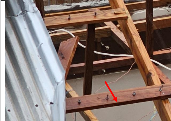
Roof sheets pulled over the screws – leaving the screws behind.
