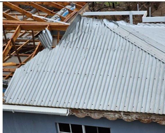
Screws spaced 150 mm (6”) apart, but cladding torn.
