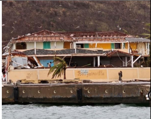
Hotel accommodation with partial roof cladding loss.
