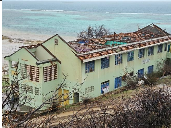
Full roof cladding and frame loss of school.
