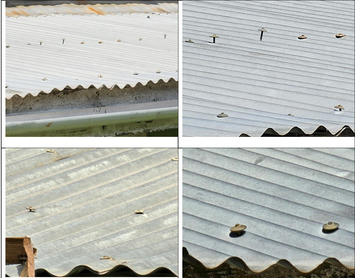
Figure 15 – Partially pulled out nails.
